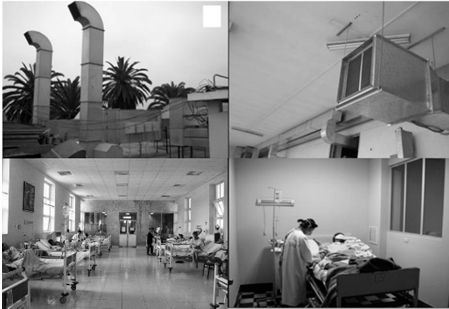
FIGURE 4. Photographs of air-elimination ducts (upper left); air-injection motor and filter (upper right); main ward with natural ventilation (lower left); respiratory isolation room (lower right).
